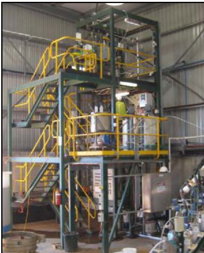
Figure 2: Continuous 4 Pot Pilot Plant.
