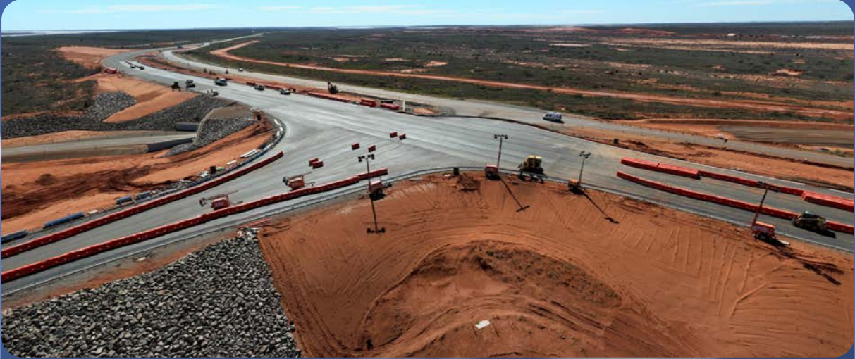
Above: Onslow/Warrida Road Intersection constructed for Main Roads WA & Mineral Resources Limited (MRL).
