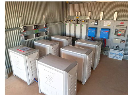
6 x ZCell Offgrid System with 20kWp solar array Regional Queensland Off-Grid House Installed in June 2017 by Offgrid Energy Australia
