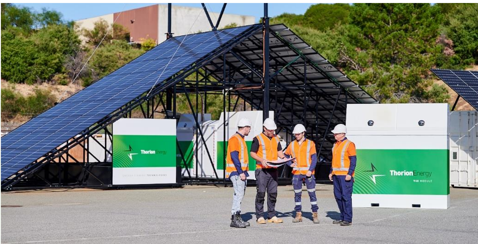
Figure 6 – Thorion standalone power system fitted with vanadium redox flow batteries
