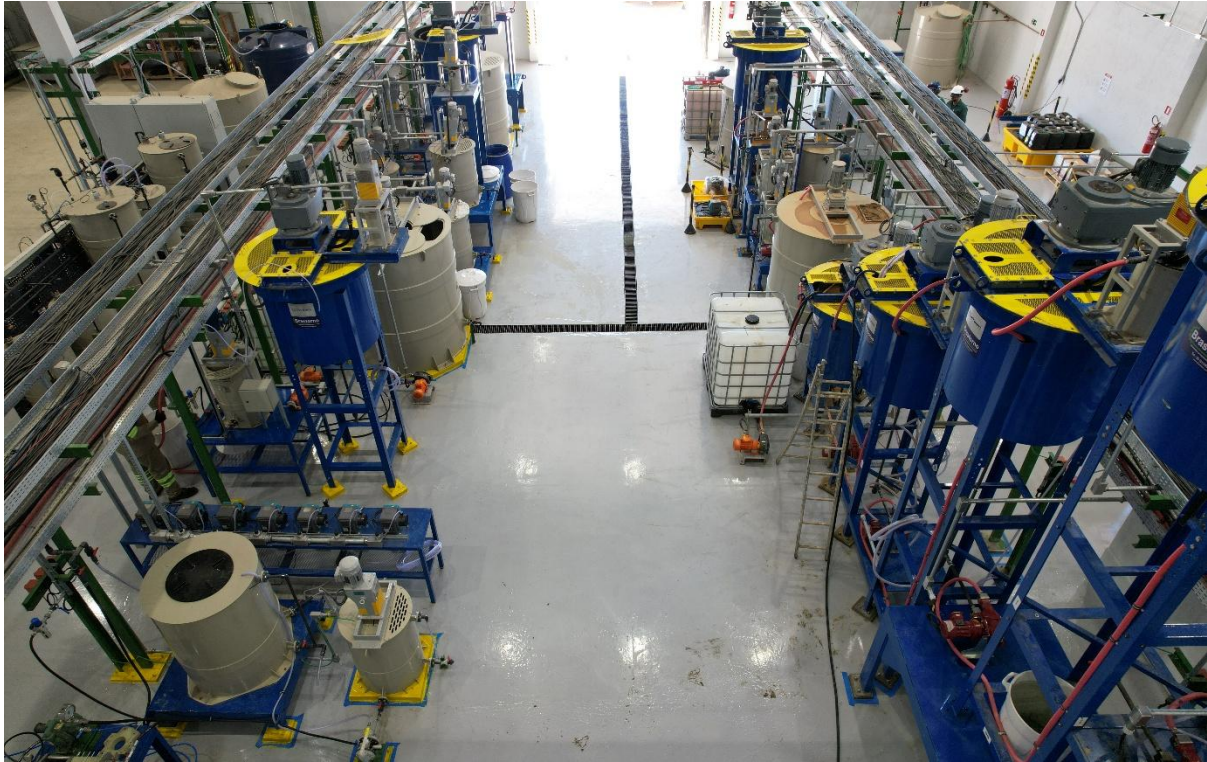
Figure 6: The Demonstration Plant replicates the Colossus project flowsheet. (Top right) Desorption stage, (bottom right) Counter Current Decantation ('CCD') stage to maximise rare earth elements ('REE') recovery and ensure spent clay meets all environmental limits for mining pit rehabilitation, (top left) Impurity removal stage, and (bottom left) MREC precipitation and filtering stage.
