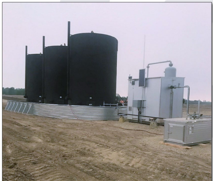
Figure 1 - Surface Facilities on the newly constructed pad at Wizard Lake
