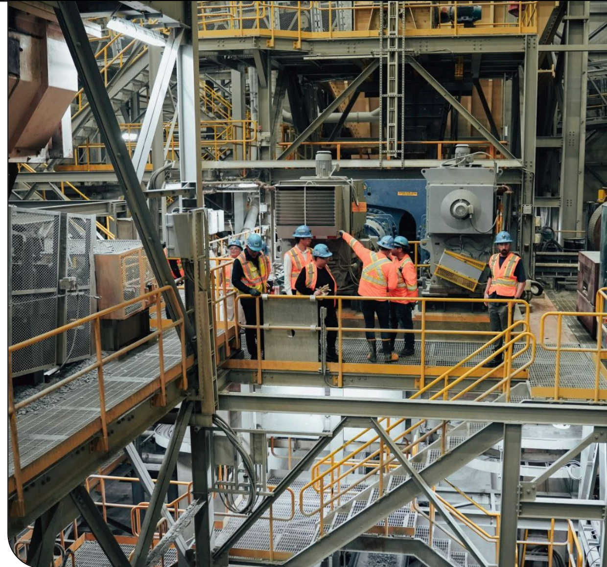
Image: Renard Dense Media Separation (DMS) processing plant (Investor Site Visit) July 2024
