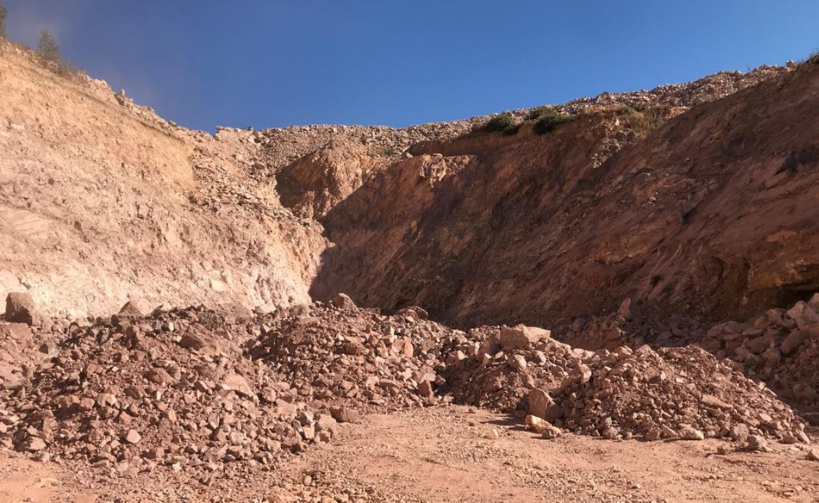
Image 2: Backfilling of Pit 3 commenced during the quarter which will complete the rehabilitation project
