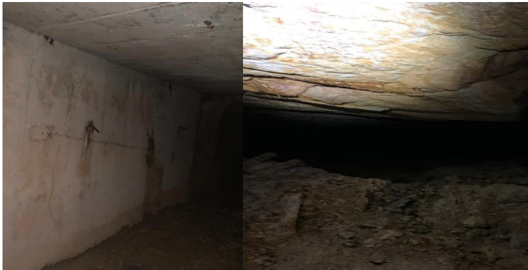
Image 4: Good condition reported of the Qala Adit shaft infrastructure (left) and the K9A hanging wall (right)
